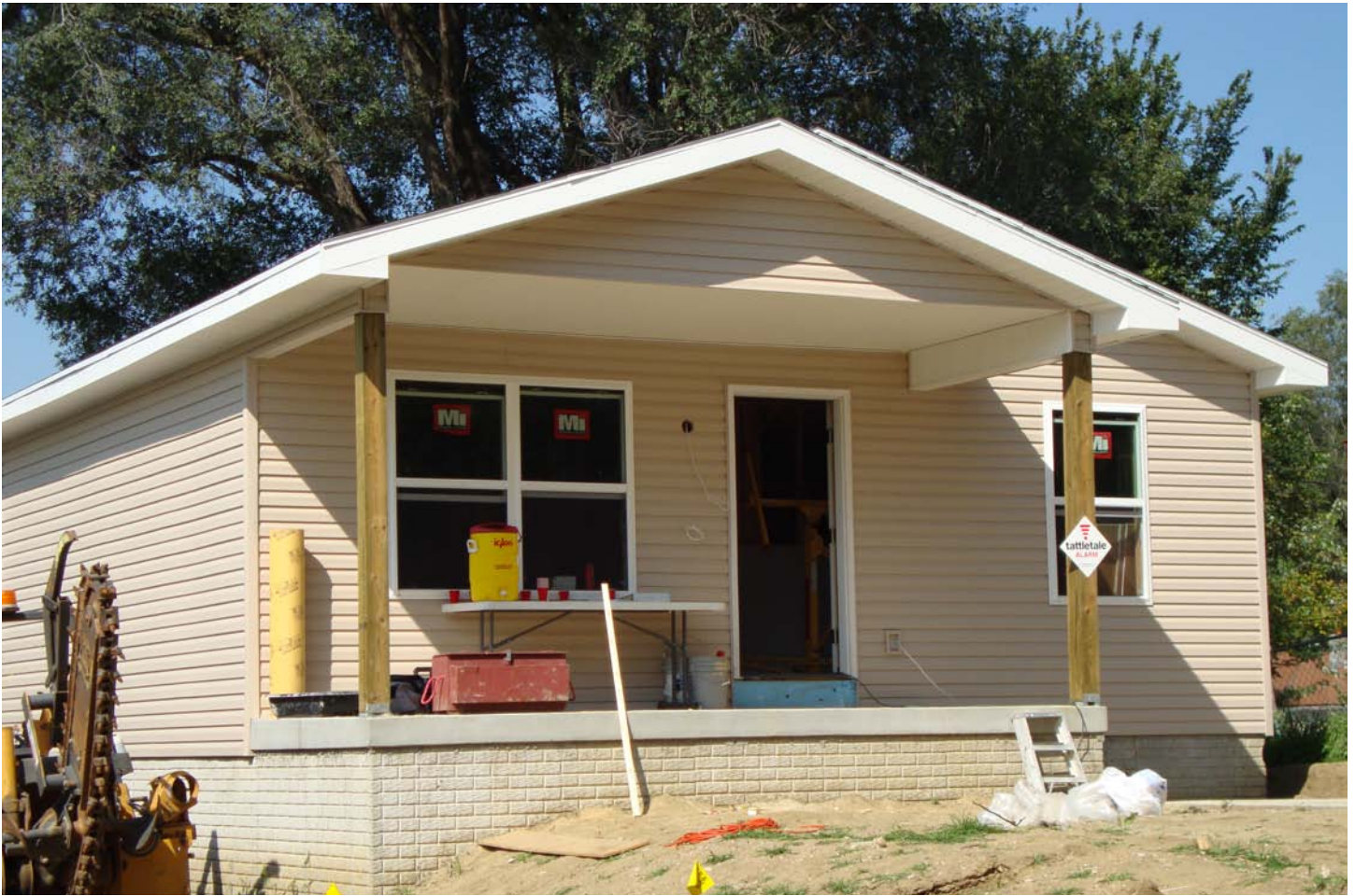
The Faithful Builders Coalition's 2009 house was built with support from Thrivent Financial for Lutherans.
